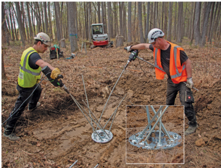
A Spinnanker crew did onsite tests, threading steel rods into a circular base, similar to ones used in the lookout tower's foundation.
